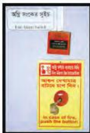
Fire Alarm Switch
