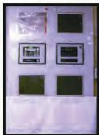
Fire control panel
