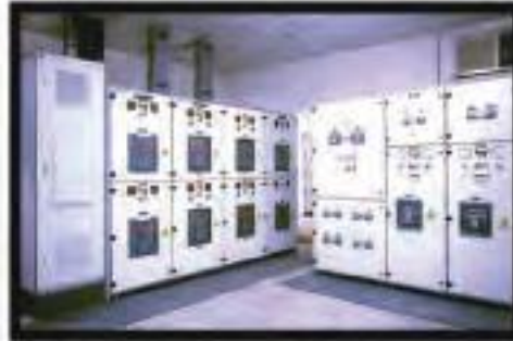
Generator control panel
